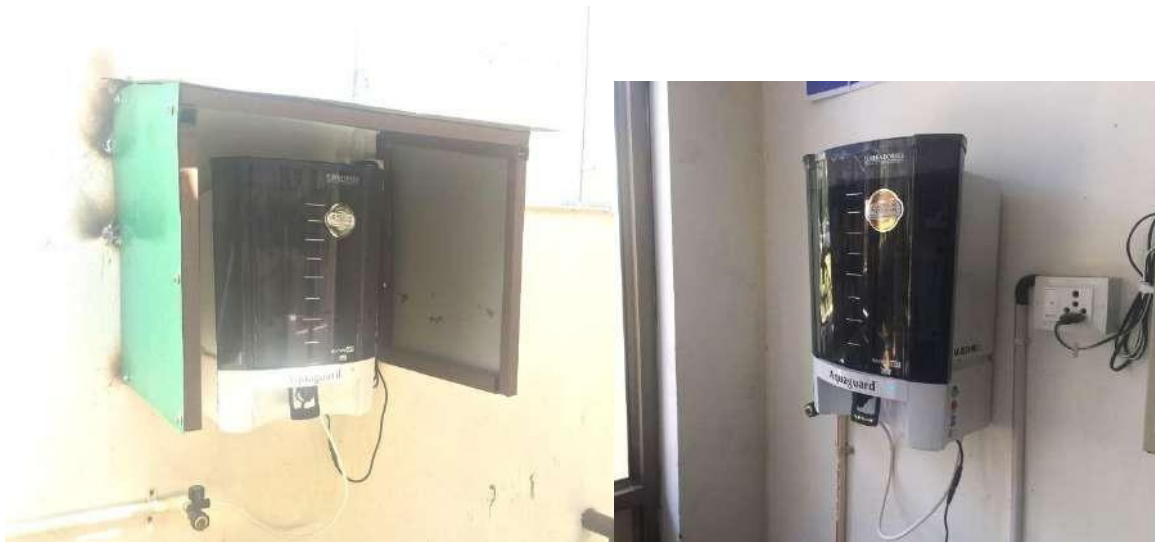
Clean and freely accessible RO water facility for staff and students
