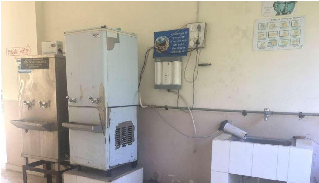
Cold RO water and washing area facility for staff and students
