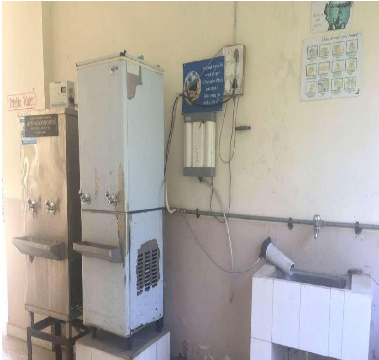
Cold RO water and washing area facility for staff and students
